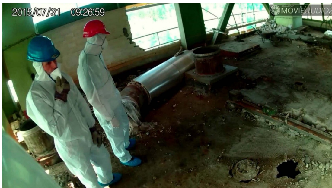
Figure 8. Uranium concentrate dryer—inside the building.
